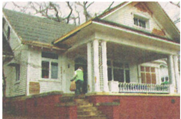
NEW HEADQUARTERS: “Green” renovation work continues at the new Upstate Forever headquarters on Pettigru Street.
